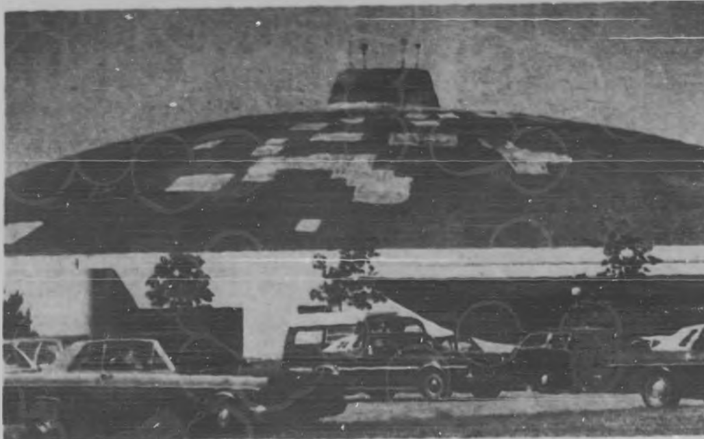
Ineffective Dome spot repairs
