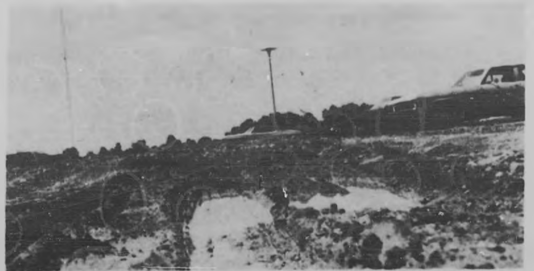
Mancating potholes in parking lot -C.
