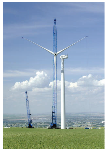
4c. Installing the blades for a 1.3 MW turbine at the Nine Canyon Wind Project (Washington, 2002).
