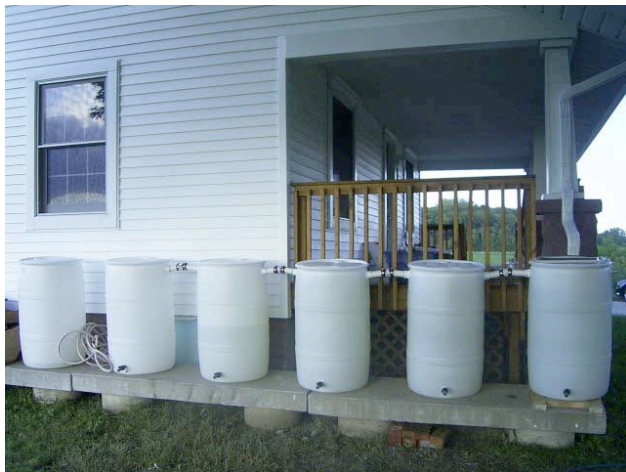
Rain barrel collection system at the community garden, along the Wesley House
