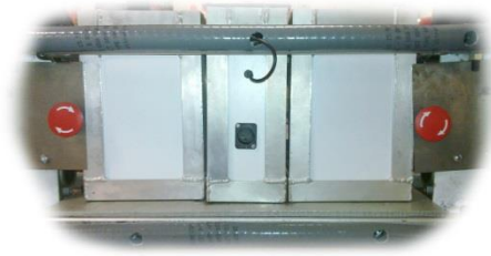
Figure 28: Emergency Stop Switches
