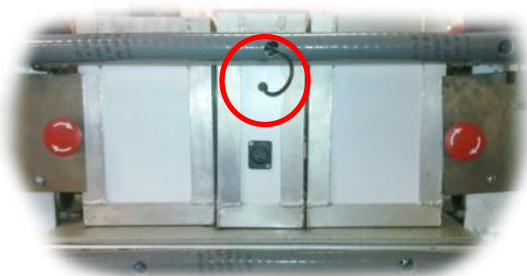
Figure 79: Emergency Stop Cable
