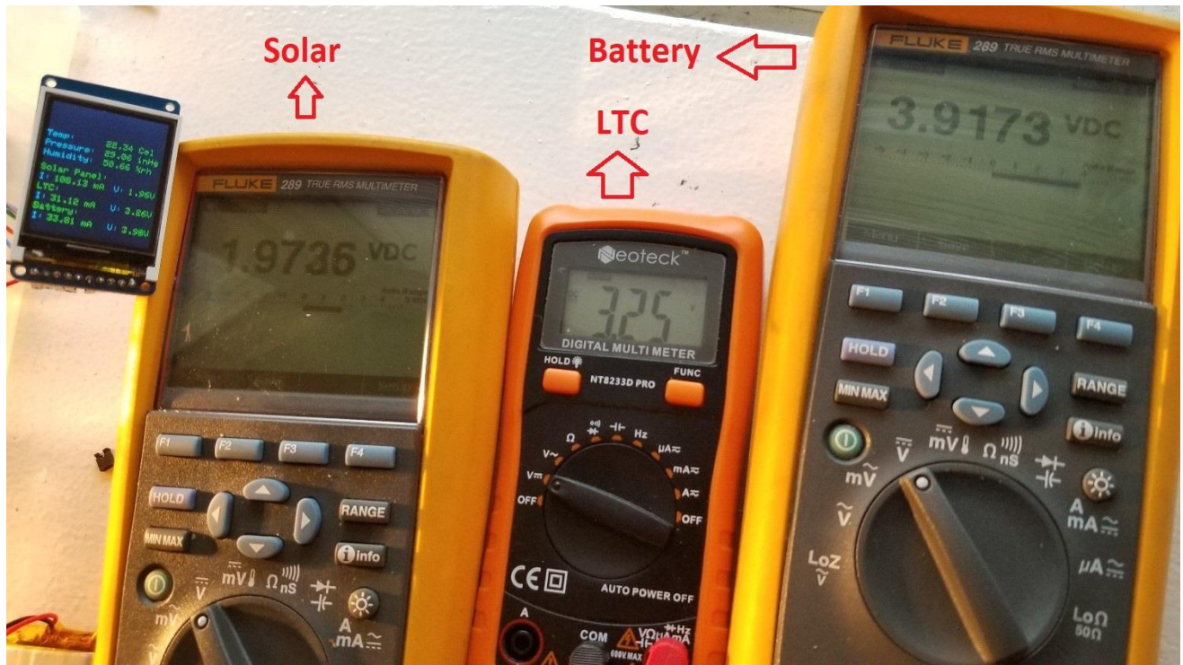
Figure 34: Voltage reading verification using multimeters
