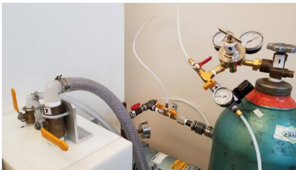
Figure 11: Actual connection of nitrogen and vacuum to the glovebox
